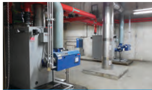
Salmon River Hatchery heating system.
